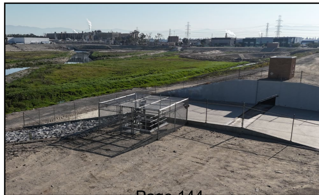
Outlet Control Gate/Rubber Dam System
